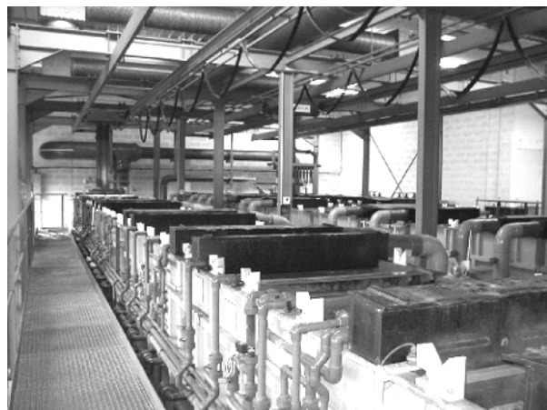
Figure 4 ; Automated chemical cleaning plant.
